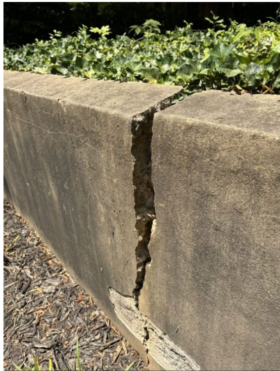
Left side wall with damage
